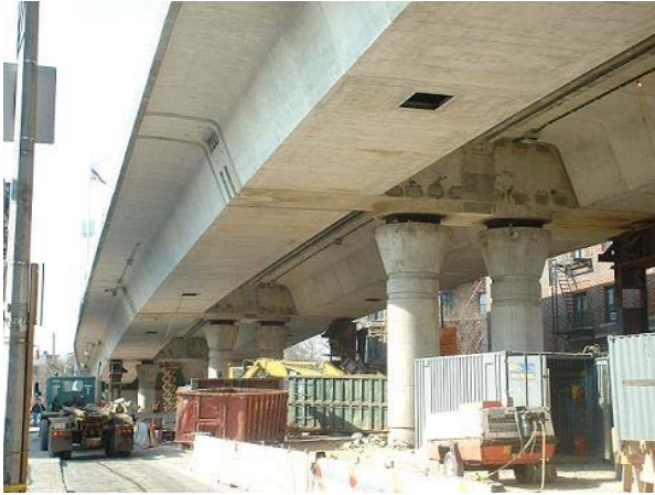
Figure 3 Adjacent box girders are connected via a post-tensioned diaphragm during the final stages of construction
